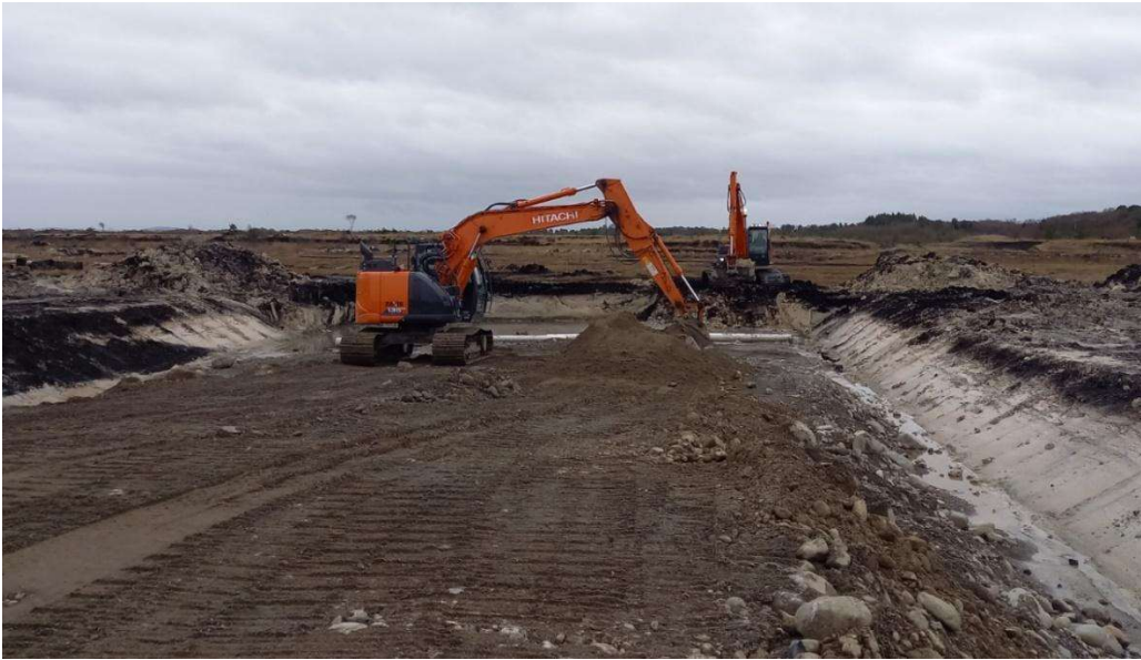
Plate 4-9 Internal roads under construction using the excavate and replace method. Source BnM.
